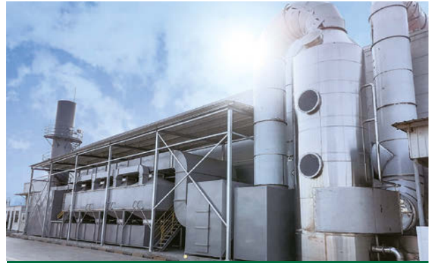
Volatile organic compound treatment facilities were employed at Greatview's Shandong Factory
