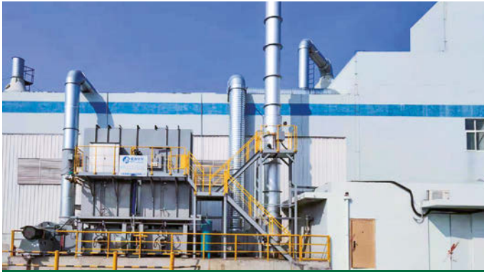
Volatile organic compound treatment facilities were employed at the Qingdao Likang Factory
