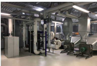
Thermal Recovery System
